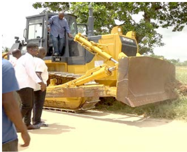
A grader commences construction works on phase two of the Goshi-Madunguni road in Kakuyuni Ward of Malindi Sub County, Kilifi County.
